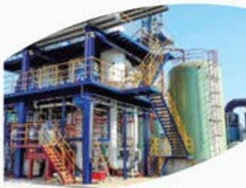
Salt Recovery Plant (SRP)
