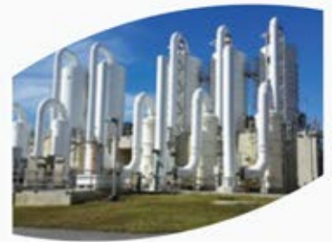
Water Treatment Plant (WTP)
