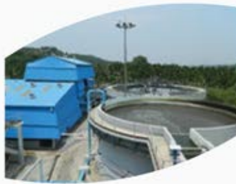
Sewage Treatment Plant (STP)
